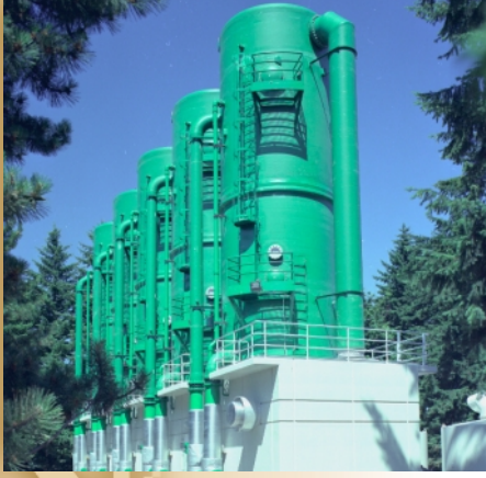
Air strippers designed and built by Ershigs for the city of Vancouver, Washington. This system is for the removal of volatile organic compounds from water.
