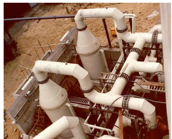
Two oxy-generators and piping delivered to Hoogovens Steelwork in the Netherlands. These generators are used to treat wastewater.
