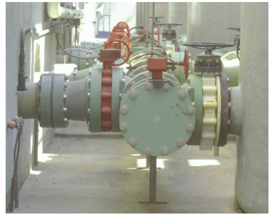
Fibercast's CL 2030 vinyl ester pipe and flanged fitting system, delivered to Gould Electronics. These components are used in their printed circuit board/electro-formed foil division.
